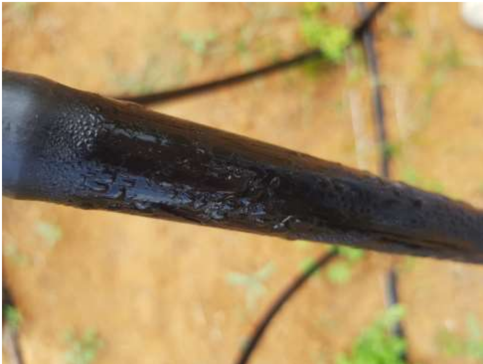
Condensation forms on the external surface of the pipes that flow by gravitation to the soil and roots.
